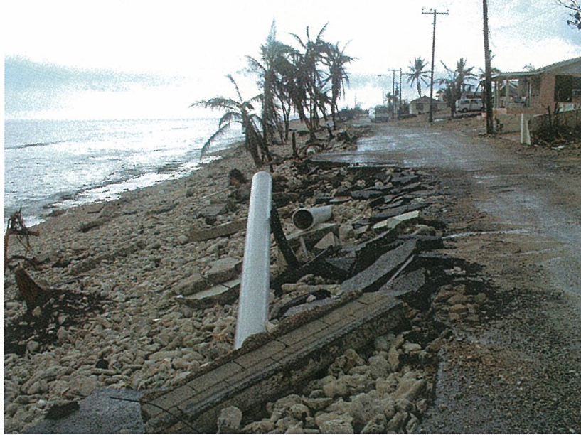
Seaview Road entrance into East End (12" main) September 2004 Hurricane Ivan Damage
