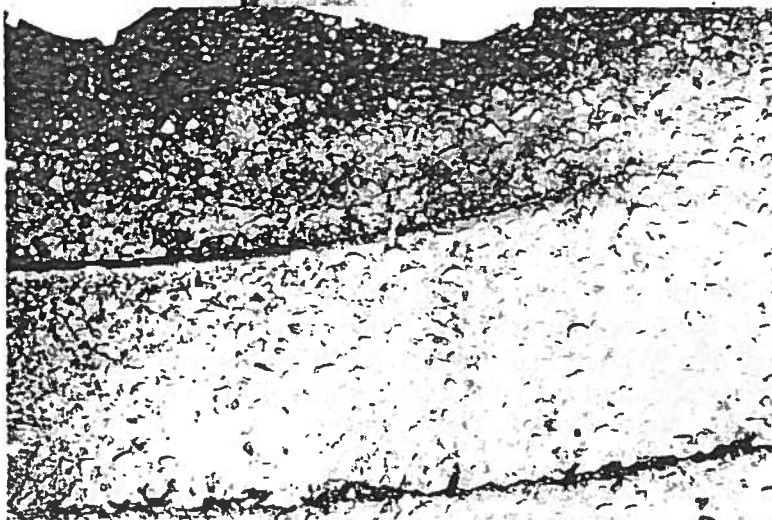
An example of the concrete corrosion of the West Bay Beach Sewerage structures
