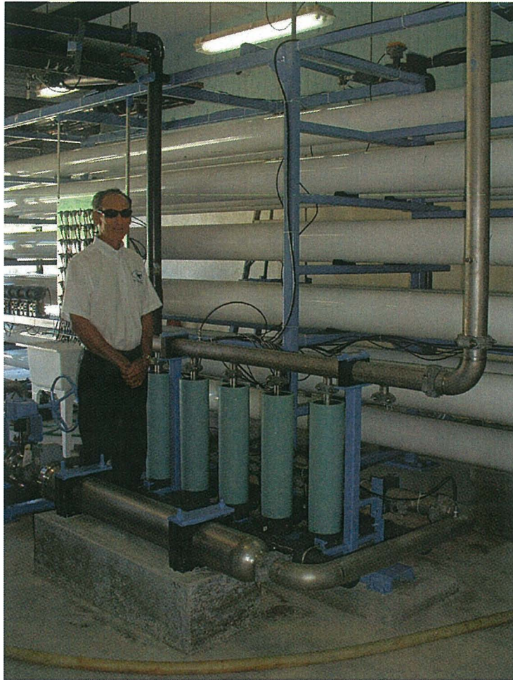
Cayman Brae RO Plant February 2003
